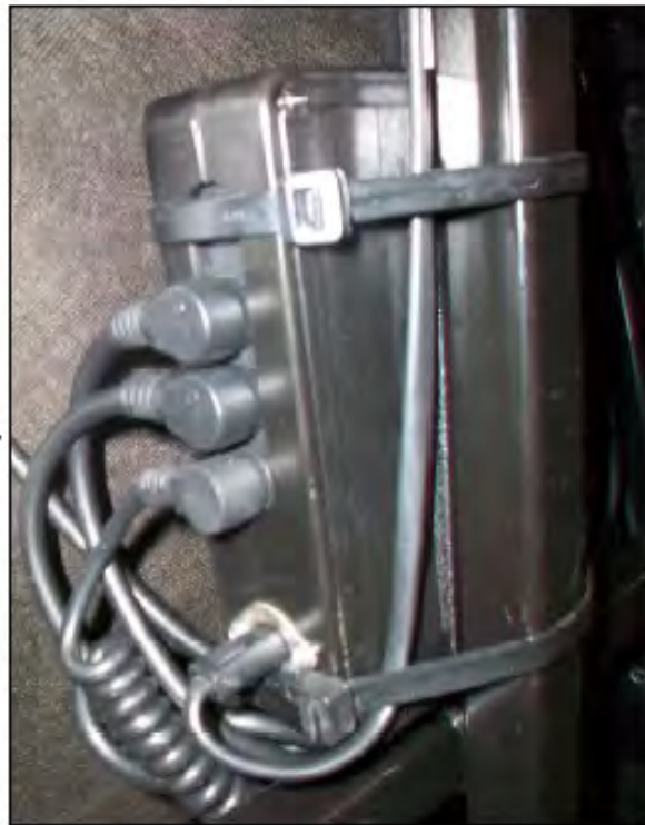
Control Box Close up View
